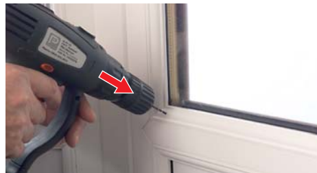
5. With the drill at 90° to the surface, drill Ø2.5mm hole 1 off on each side
